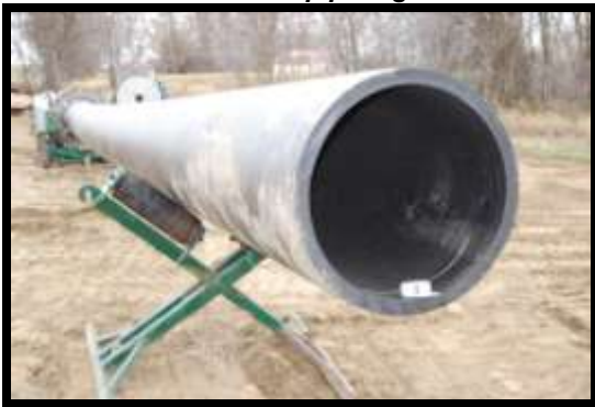
2-ft I.D. High-Density Polyethylene (HDPE) piping
