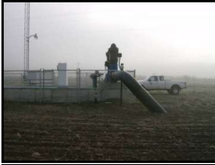
New Touchet Westside/Eastside Irrigation District pumping station
