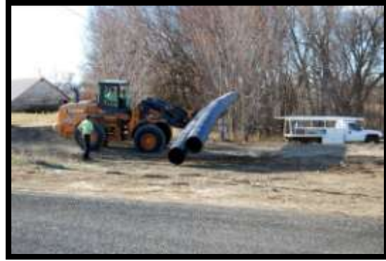
Staging HDPE piping used to go through stand of trees and under county road
