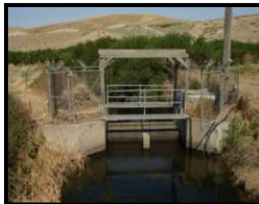
Non-compliant fish screen at Hofer dam
