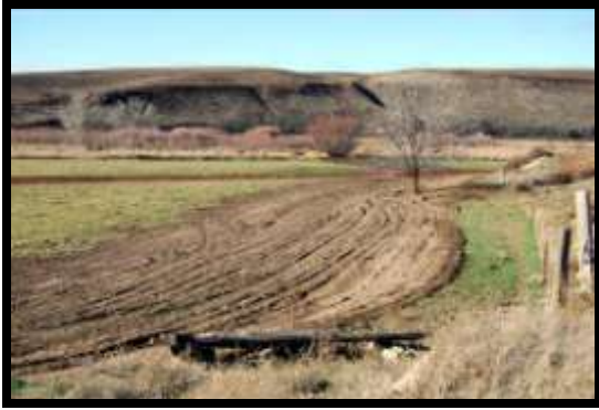
Old Eastside Canal after being filled with soil and new pipeline alignment in background
