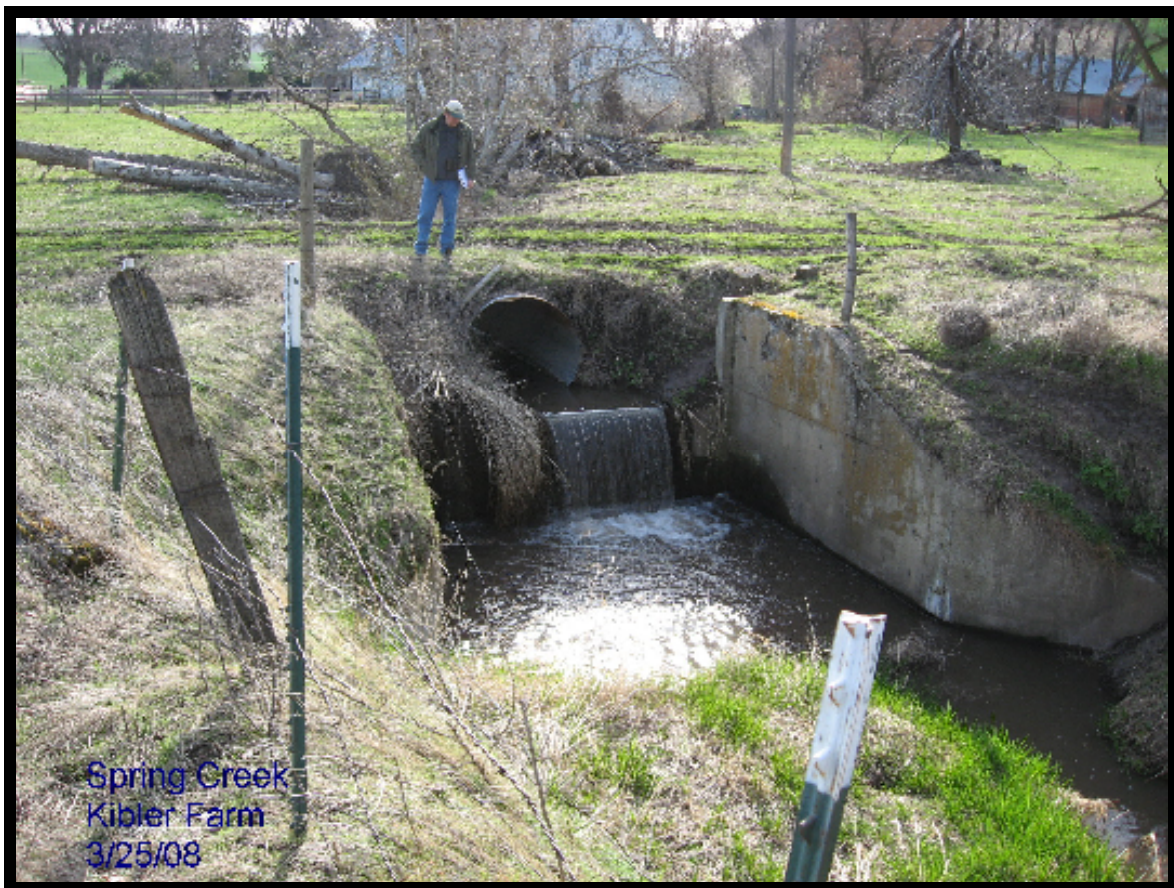
Figure 2: Perched culvert and gully plug structure at Margaret Kibler Farm prior to project construction
