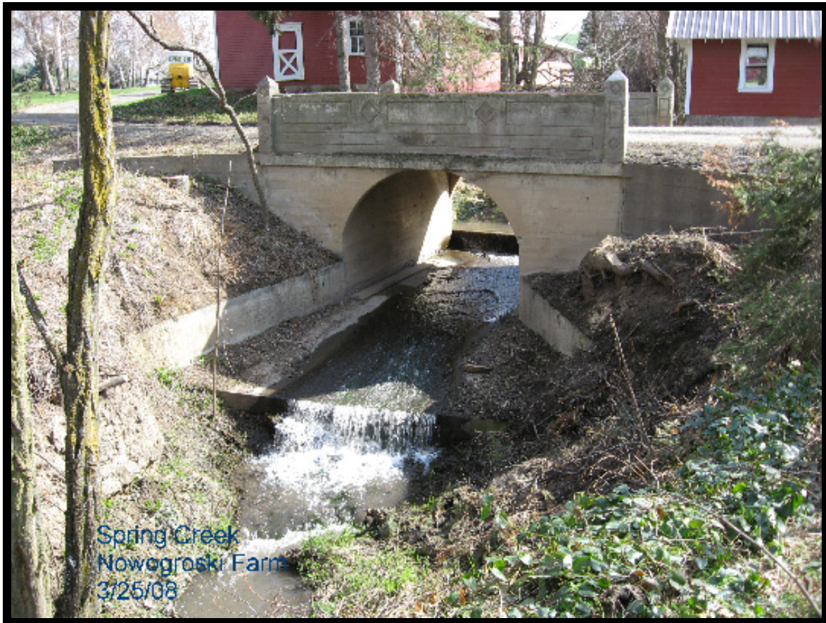
Figure 1: Nowogroski headquarters bridge and perched outfall apron – the lowest barrier to fish migration on Spring Creek prior to the project construction.
