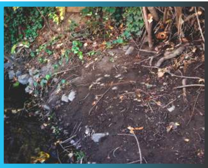
Area prone to erosion
