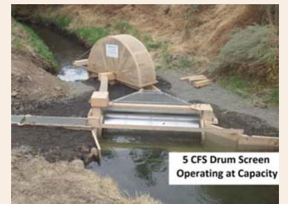
Titus Creek Fish Passage and Screening project after construction. Reduced ESA listed fish mortality from irrigation diversion and stranding.
