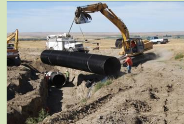
A 48-foot long section of 66-inch diameter HDPE irrigation pipe gets placed in the trench
