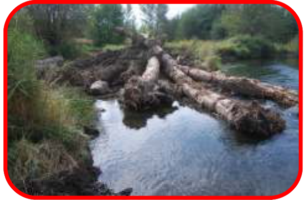
APEX LOG JAM USED TO INDUCE FLOOD-PLAIN RE-CONNECTION ON THE MCCAW PROJECT, TOUCHET RIVER, 2013
