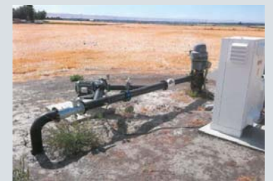
The landowner became compliant with state metering laws when he updated his pump station to the 21st century and added a magnetic flow meter.
