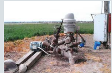
Pump station before — no water meter and out of compliance.
