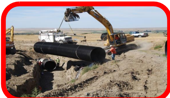
Installing 66-inch pipe for the 2,800 ft. phase of the GFID North Lateral in 2013
